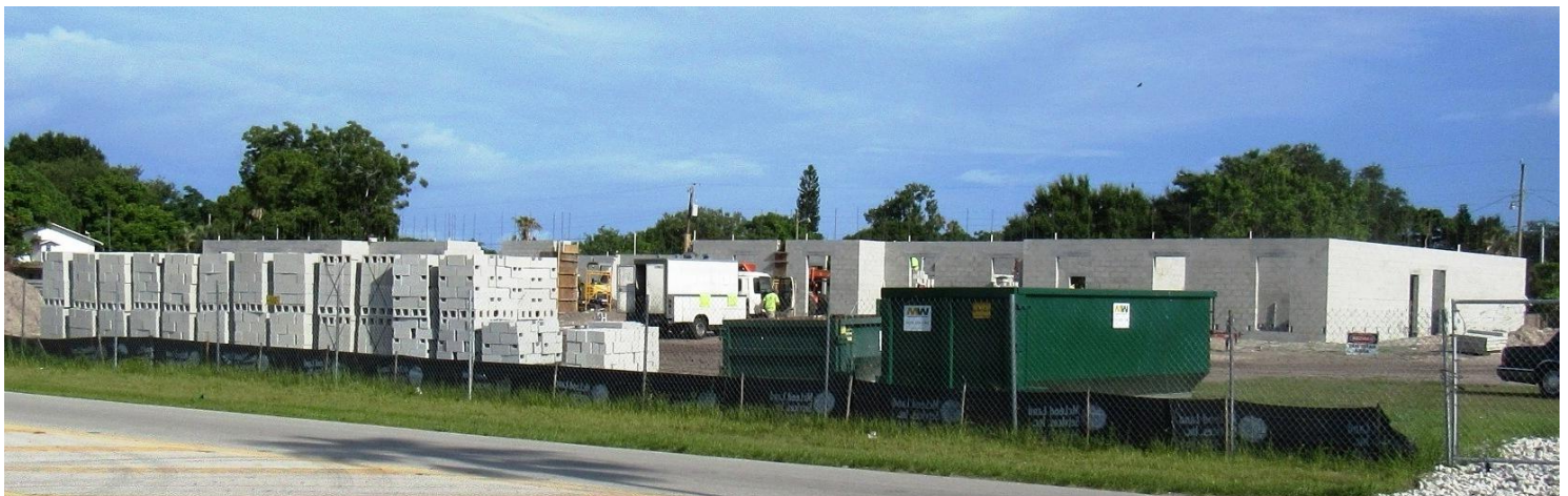
Home2 Suites by Hilton being constructed on Albee Road at Tamiami Trail in Nokomis
